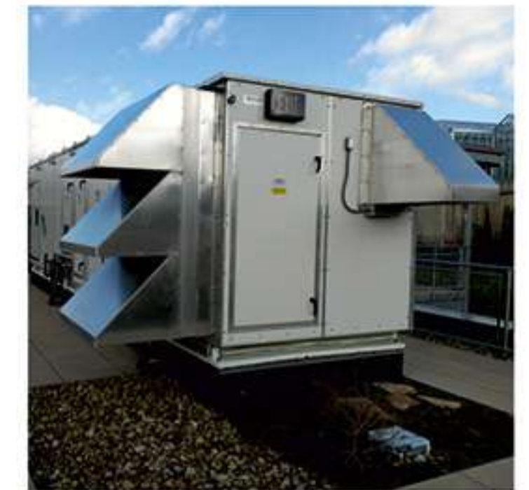
• Energy Recovery System
